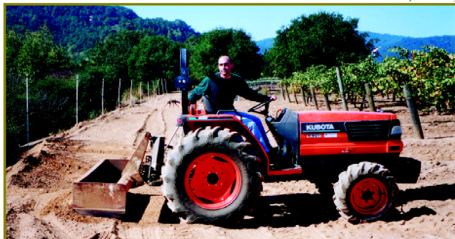
Solis Winery production manager Mike Vanni works on building a berm that will help prevent silt and pollutants from washing into the creek.
