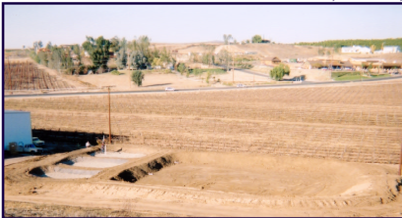
Shown under construction are Maurice Car'rie Winery's three settling ponds and a spreading basin for process water with wetlands habitat. The system is now nine months old.
